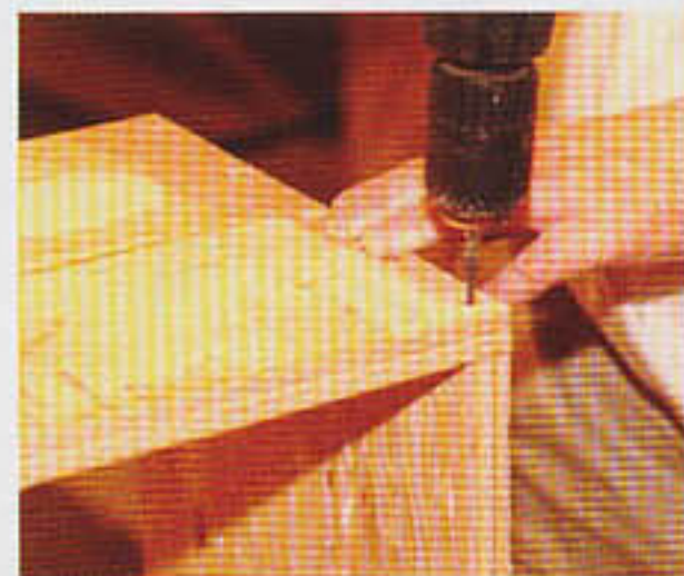
06 Plasterboard screws are perfect for screwing ply as they do not split the veneers and the hold is excellent
