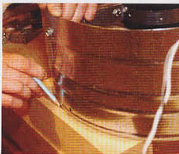
09 The fan is held in place with blocks, mark the radius directly from the fan housing
